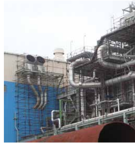
Tata BlueScope Steel's ZINCALUME® steel Jacketing of over 3.5 lakh sqm of piping and equipment at Jamnagar Refinery
