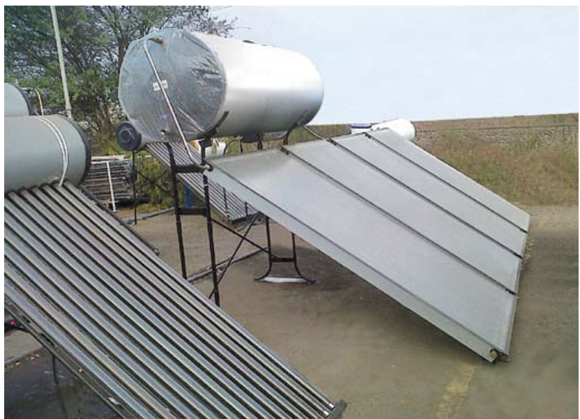
Solar Water Heaters
