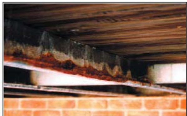
Figure 1: Example of corrosion that results from contact of CCA treated timber with galvanised purlins.
