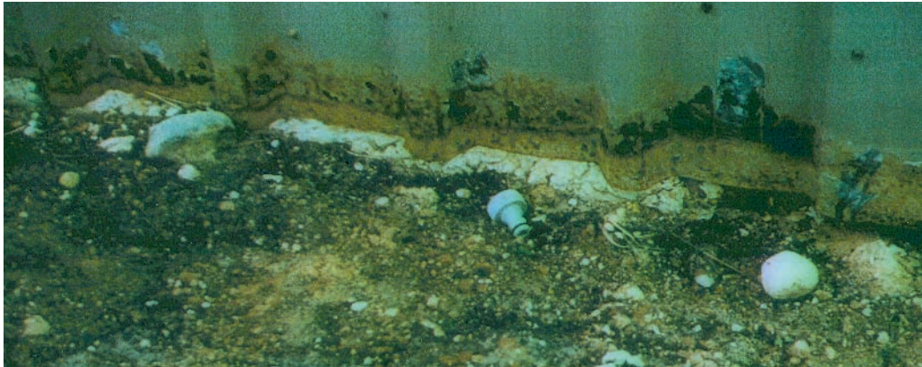
Figure 1: Immersed Shed Wall
