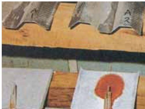
1 Aluminium to ZINCALUME® steel gutter ( left ) Aluminium to zinc-coated ( galvanised ) gutter ( right )
