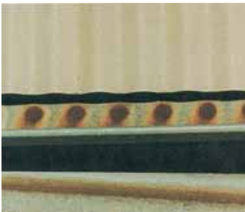
Early failure of zinc-coated gutter receiving water from pre-painted zinc-coated steel roof.
