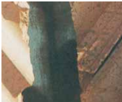
Typical early failure of zinc-coated gutter receiving water from terracotta roof.
