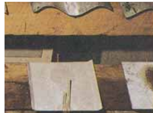
4 Zinc-coated steel to ZINCALUME® steel gutter ( left ) Zinc-coated steel to zinc-coated steel gutter ( right )
