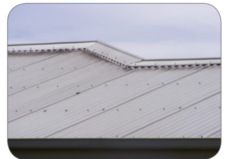
Figure 3: Photograph of a roof made from COLORBOND® steel showing isolated fungal growth in the vicinity of the ridge capping.
