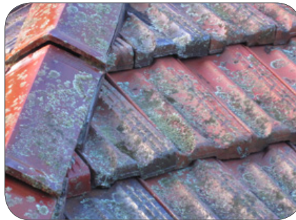
Figure 1: An example of lichenous growth across the surface of a tiled roof.
