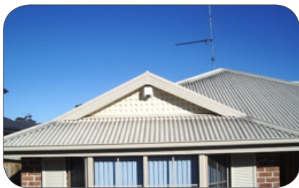
Figure 5: Photograph of a roof made from COLORBOND® steel showing uniform coverage of fungus. By way of comparison, note that the body of the roof was supplied in the same colour as the gable detail.
