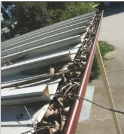
1) A typical suburban gutter clogged with leaf litter prior to cleaning.
