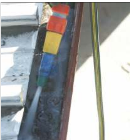
4) Spray the gutter & downpipes with water to soften and break up the dirt.
